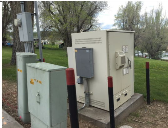
Photograph 26: Signal box located near the southwestern corner of the property, adjacent to the southern property boundary.
