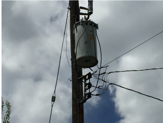
Photograph 16: Pole-mounted transformer located near the western property boundary, south of the Quonset.
