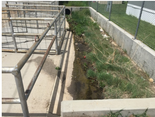
Photograph 23: Water and vegetation are visible in the storm drainage area located along the eastern property boundary, adjacent to the Livestock building depicted in Photograph #22.
