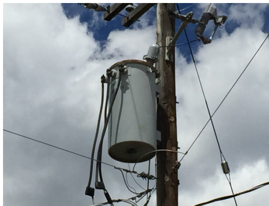
Photograph 20: One pole-mounted transformer located near the northeast corner of the parking lot, northwest of the grandstands.
