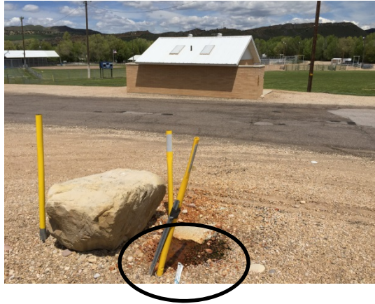
Photograph 10: Artesian well (circle) located near the southern property boundary, near the southeast corner of the property.
