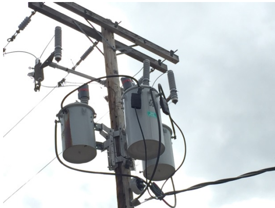
Photograph 24: Three pole-mounted transformers located near the southeastern corner of the property, adjacent to the southern property boundary. Note the green “no PCBs” sticker on the central transformer. The left transformer has noticeable rust staining, but the case is otherwise intact and leaking was not observed.
